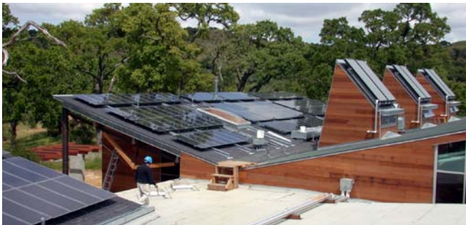
Fig. 3 East wing roof PV array and light monitors.
