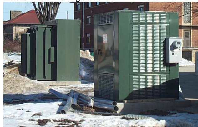
Figure 6. Photograph of electric enclosures on west end of ESC showing meter (foreground) and 500 kVA building transformer (background).
