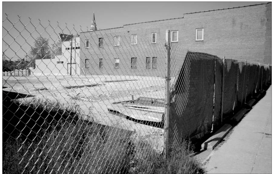
East College Street Progress: This recently-taken photo shows the most current stage of demolition on Oberlin alumni's local green building project. (Photo by Chris Hamby)
