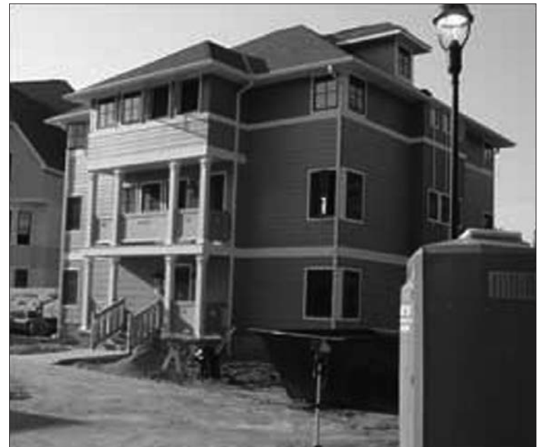
New Union Housing: Construction on the new college housing stretched into the fall move-in date. (Photo by EmilyKate McDonough)
